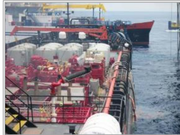
Pumping equipment installed on the deck of the HOS Centerline for BP's Operation Top Kill
